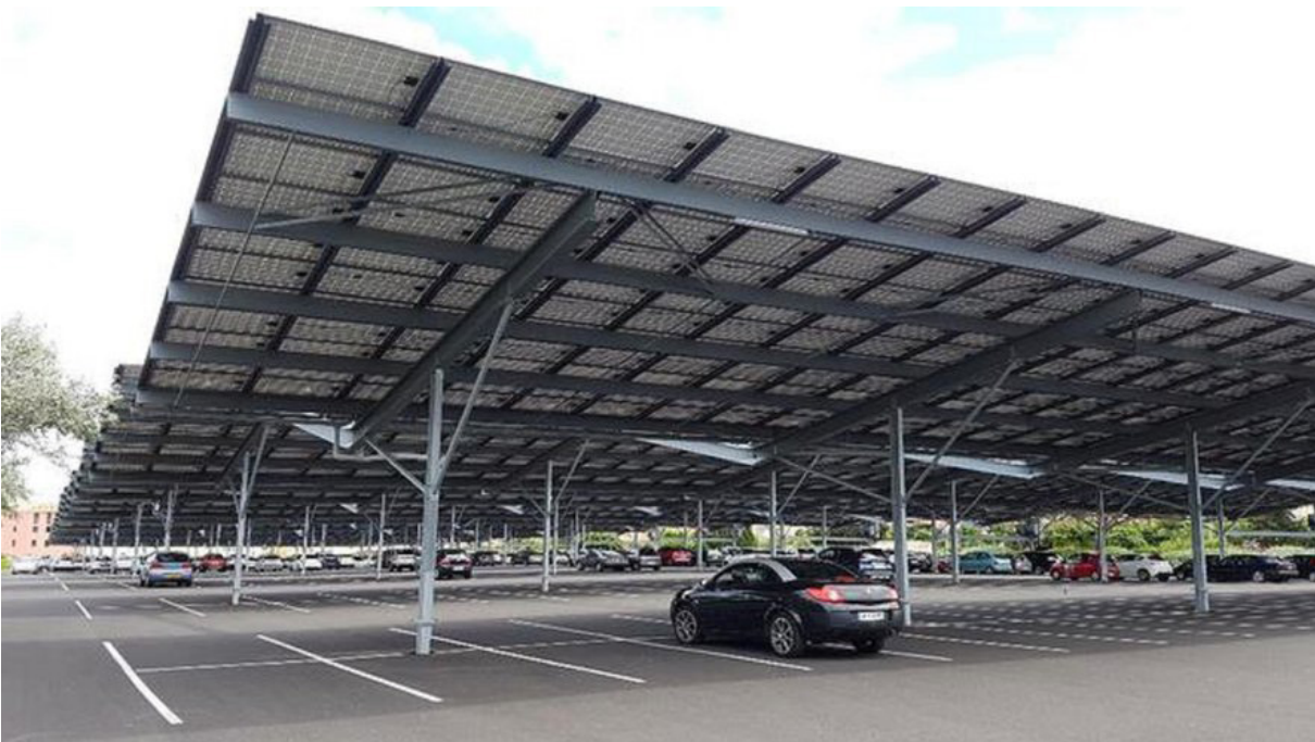
Ombrières photovoltaïques | Structure type acier
